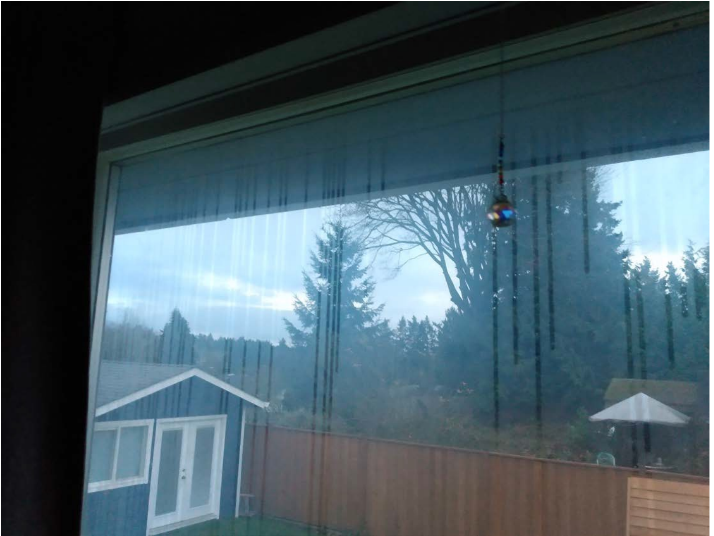
This is a very common problem. This is not condensation. It is active water leakage between window panes and onto sill and into interior space.
