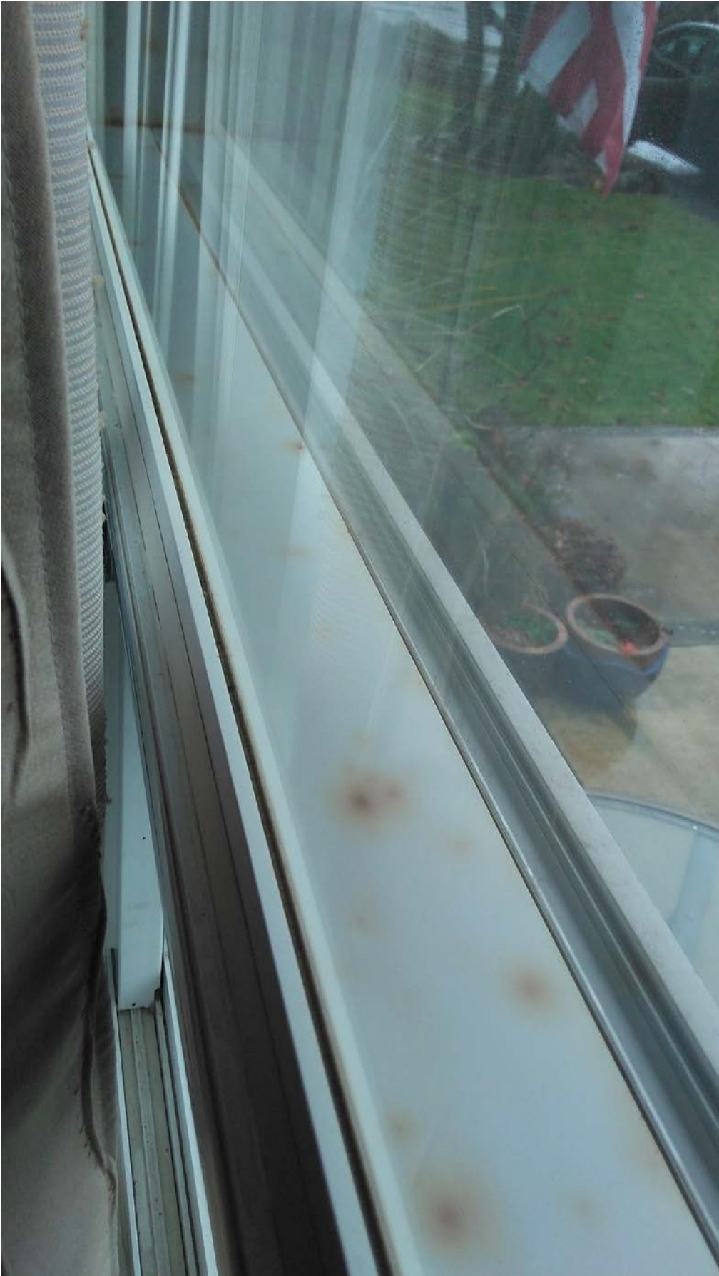
This kind of brown mold spotting is another common variant that will appear on every window in the home. It cannot be cleaned as it is imbedded into the window.
