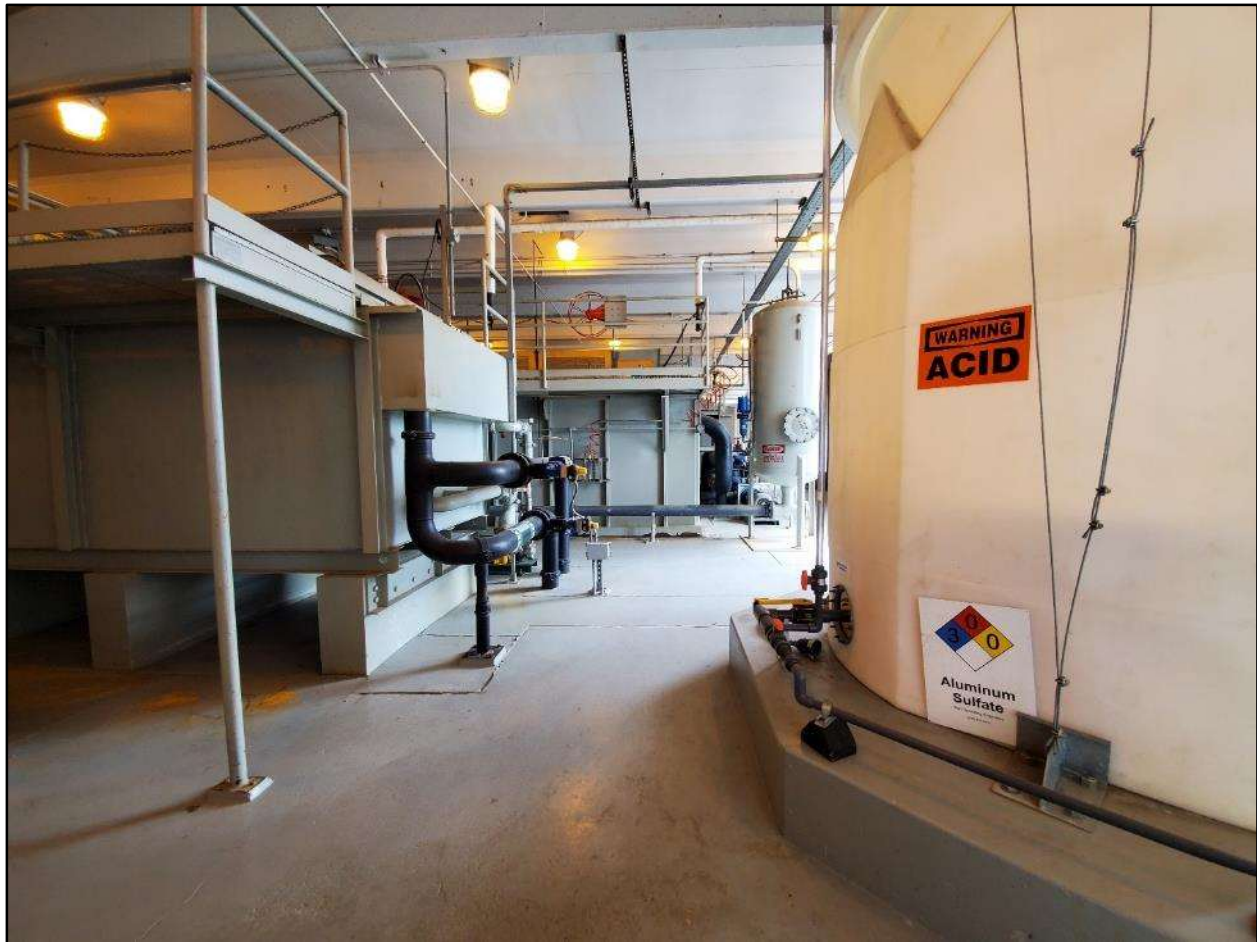
Figure 4: Existing DAF Units #1 and #2 with Alum Tank
