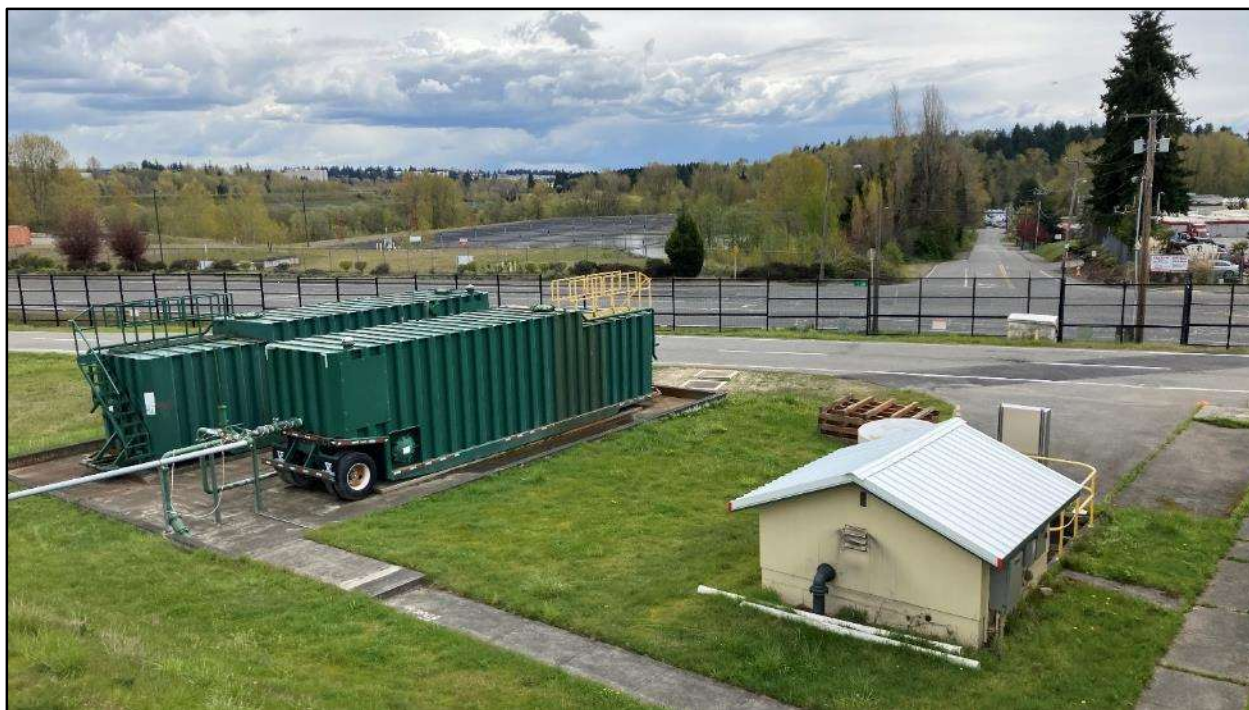
Figure 5: Existing DAF Solids Handling System
