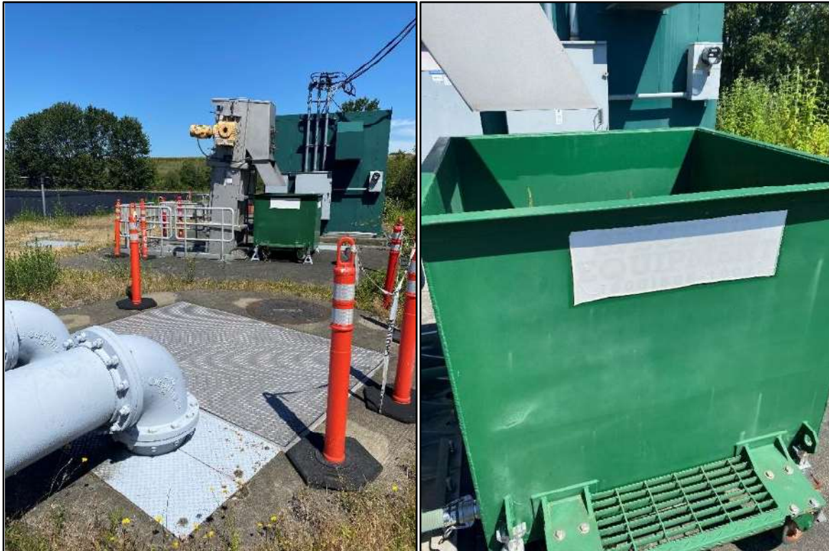
Figure 11: Photos of TS-3000 (left) and Dewatering Bin (right)
