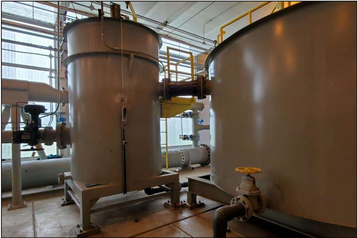
Figure 19: Existing Flash Mix Tank and Flocculation Tank
