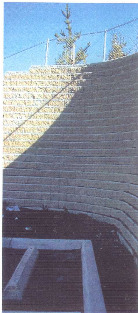
The wall itself appeared largely intact. Moisture was observed seeping through the wall, shown here. A slight bulge was observed at the top of the wall, about half of the width of the wall. (N47.22452° W122.4667°)
