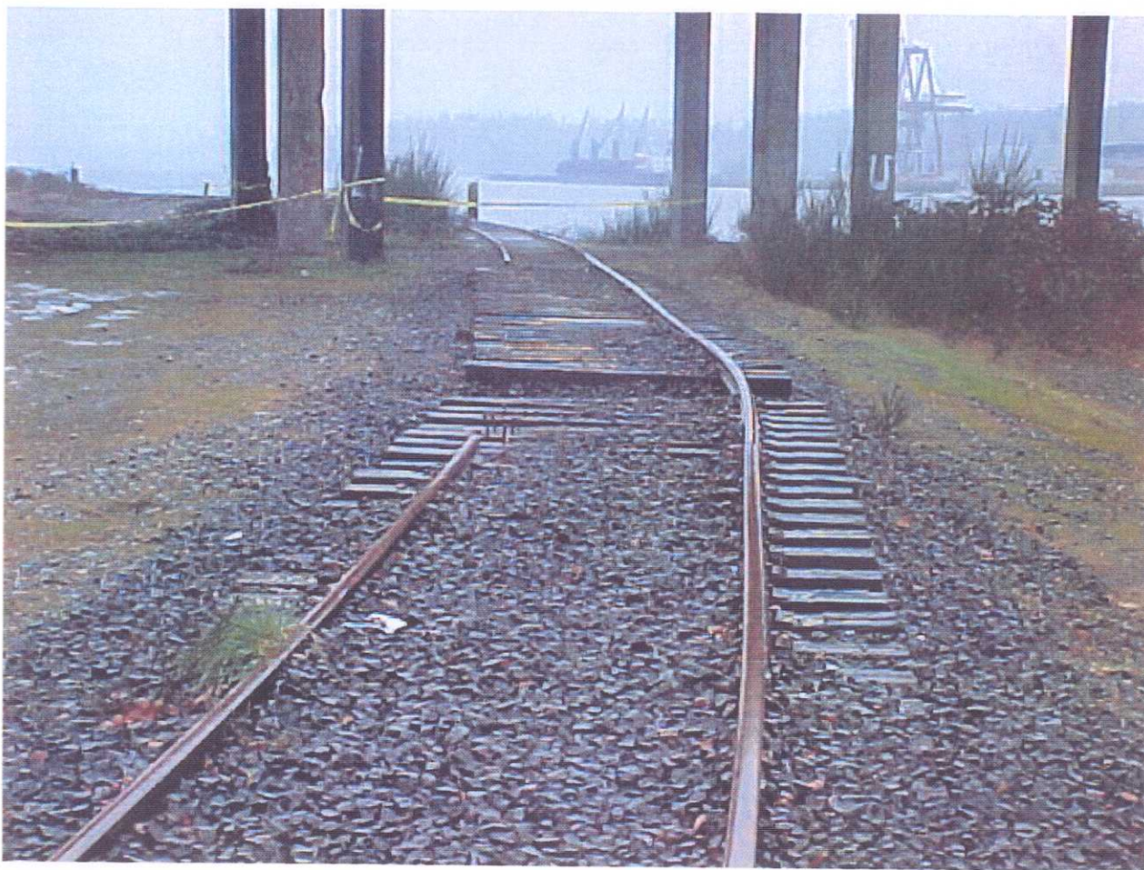
Broken rail line along the western shore of Capital Lake in Olympia (GPS N47.04401° W122.91071°; 1200 03/01/01).
