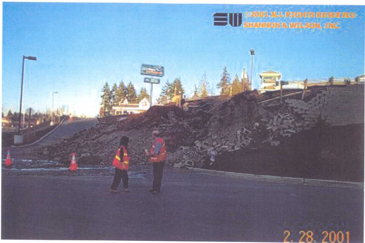
Along the right hand edge of the wall, the height of the wall was 15 20-cm high blocks for a total of 3 m (GPS N47.02479 W122.92230; 02/28/01).
