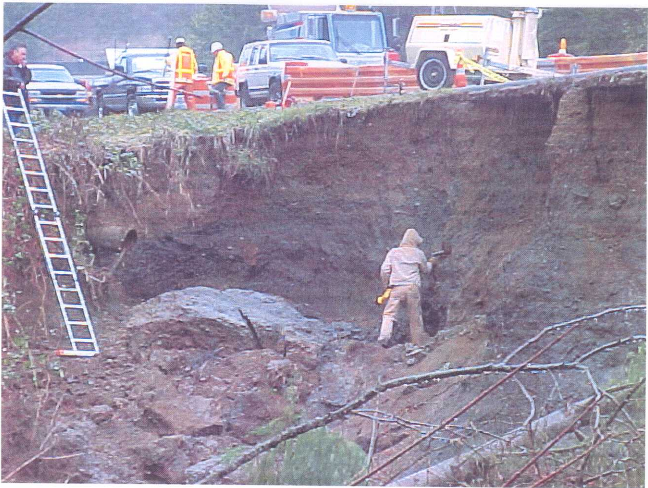
View of eastern end of the headscarp at the Highway 101 road embankment slide shown in the previous photograph. In this area the headscarp is approximately 6 m high (GPS N47.05834 W123.01365; 1050 03/01/01).
