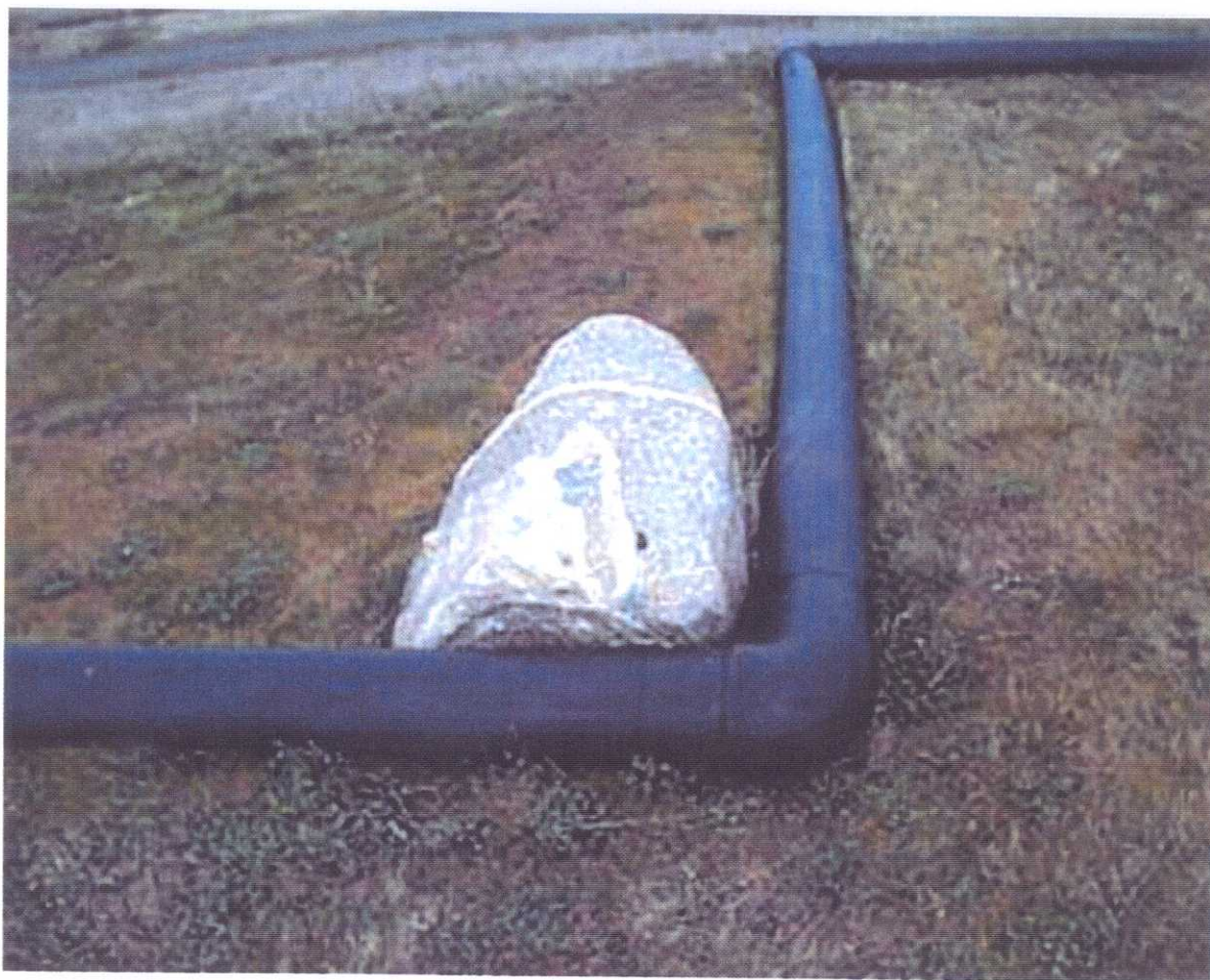
Along the north end, a boulder rested against the HDPE gas collection pipe (GPS N47.38043 W122.29422; 1215 03/03/01).
