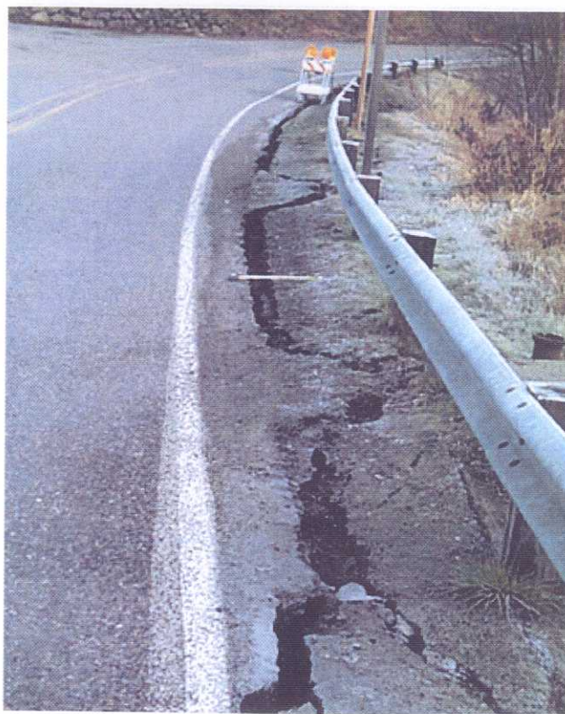
Ground cracking with outward movement of roadway edge and guard rail. Lateral offset is on the order of 18 cm. (GPS N47.1923° W122.5739°; 0745 03/04/01)
