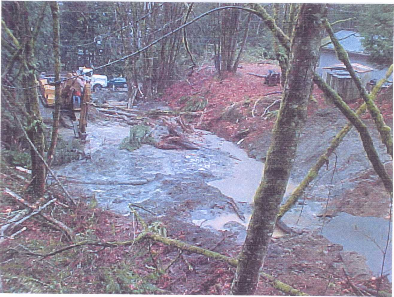
View of run-out of slide material downslope from the Highway 101 earth embankment slide.(GPS N47.05834 W123.01365; 1100 03/01/01).
