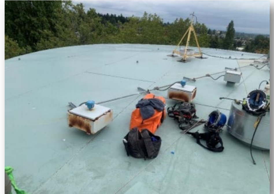
Telemetry boxes Deteriorated coating
