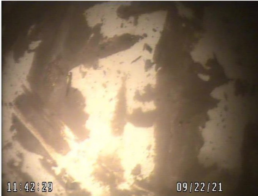
Significant rust on interior tank surfaces
