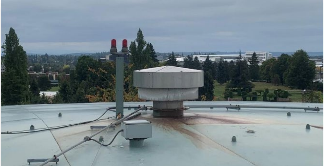
Cap Vent Moderate rust needs removal
