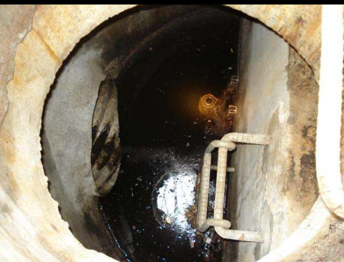
Storm water and storm drain solids
