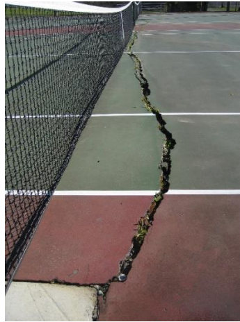
Figure CCR-7: Damage from 2001 Nisqually Earthquake to Sacajawea Park Tennis Courts
