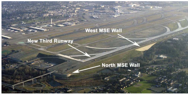
Fig. 1. Perspective aerial photo of the new third runway at STIA viewed from the northwest and showing the north and west MSE walls
