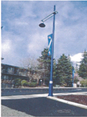
Parking lot lighting
