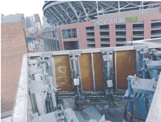
Screening of roof-mounted antennas, and equipment should be integrated into the design of the building
