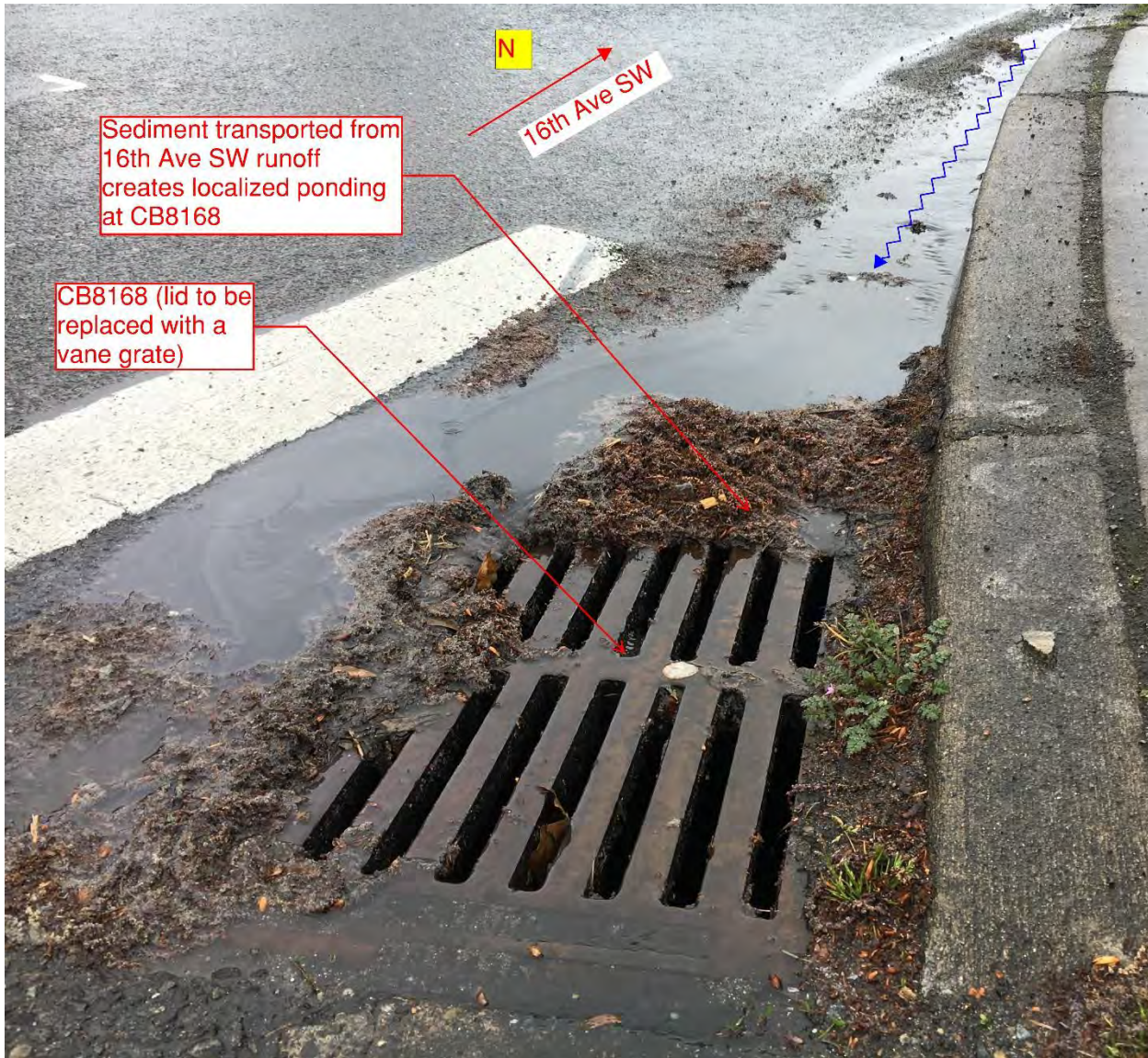
FIGURE 1: Localized ponding around CB8168 during small precipitation event. Photo date 4/8/2019, photo taken facing northeast
