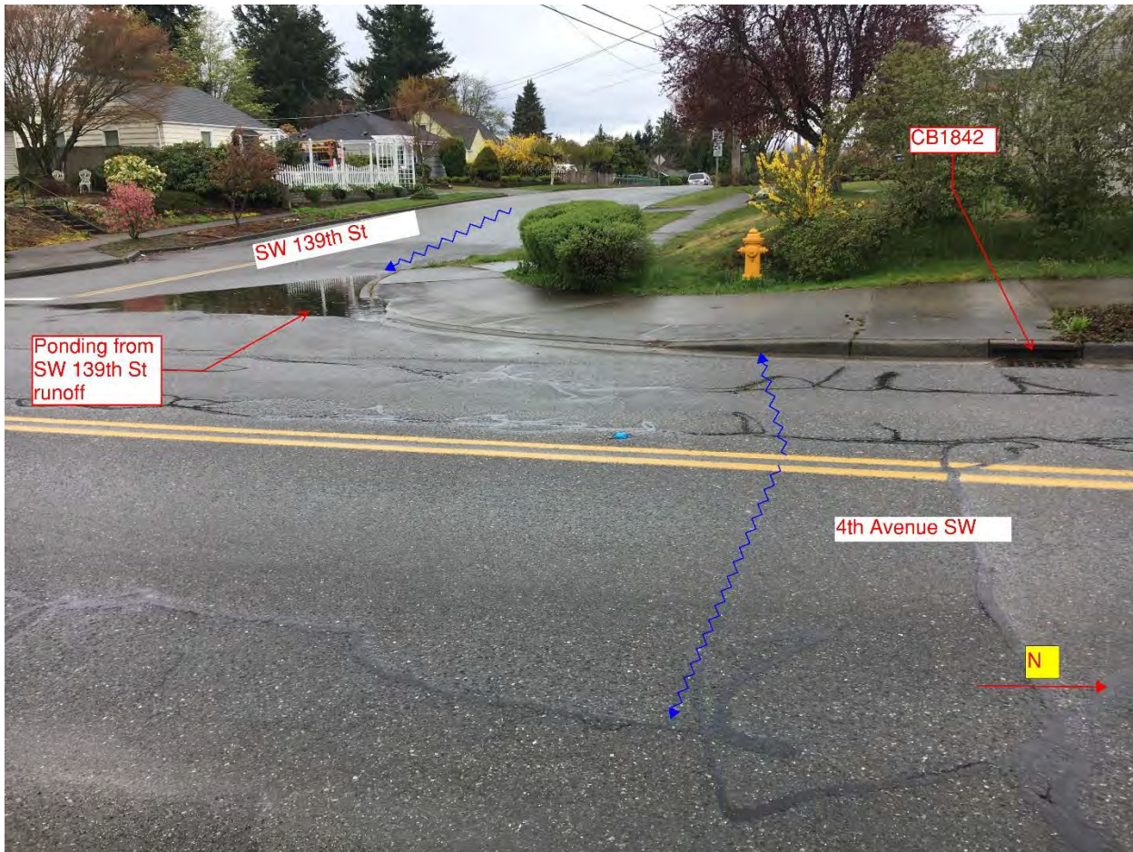
FIGURE 3: Ponding at NW corner of SW 139th Street and 4th Avenue SW. Photo date 4/8/2019
