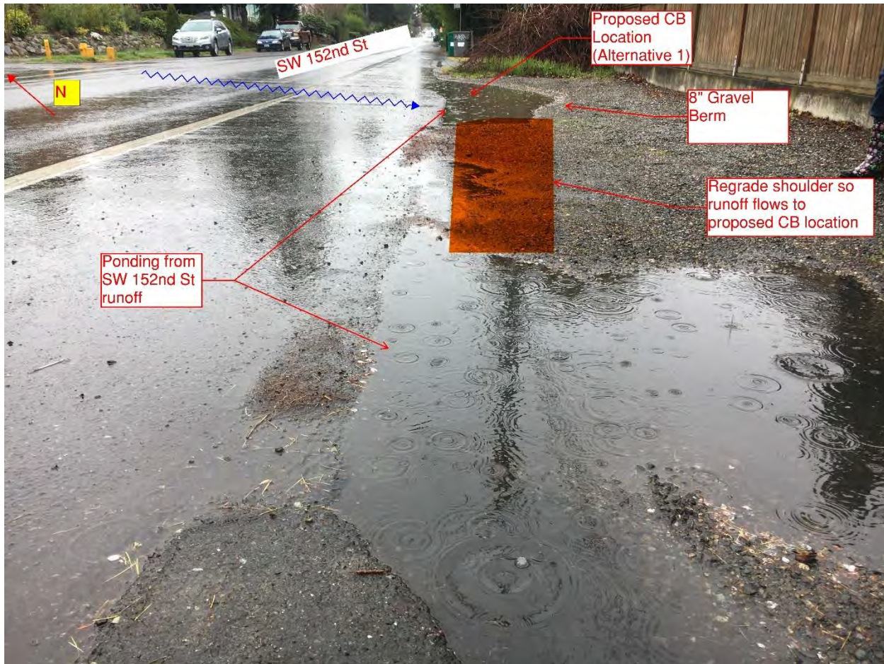
Figure 1: Ponding in south shoulder of SW 152 nd Street and 16 th Avenue SW intersection. Photo date 4/8/2019
