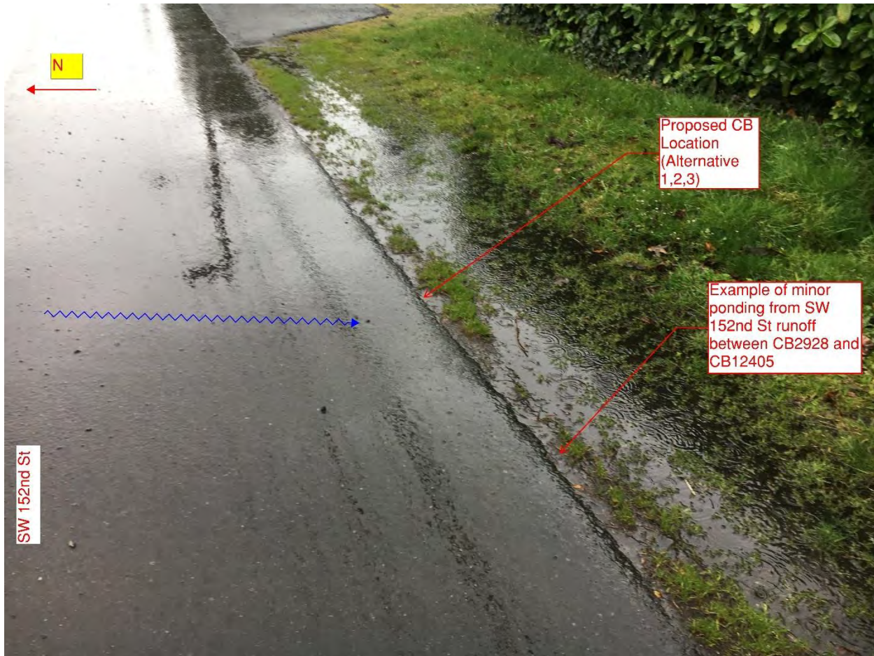
Figure 2: Small localized ponding in south shoulder of SW 152 nd Street. Photo date 4/8/2019
