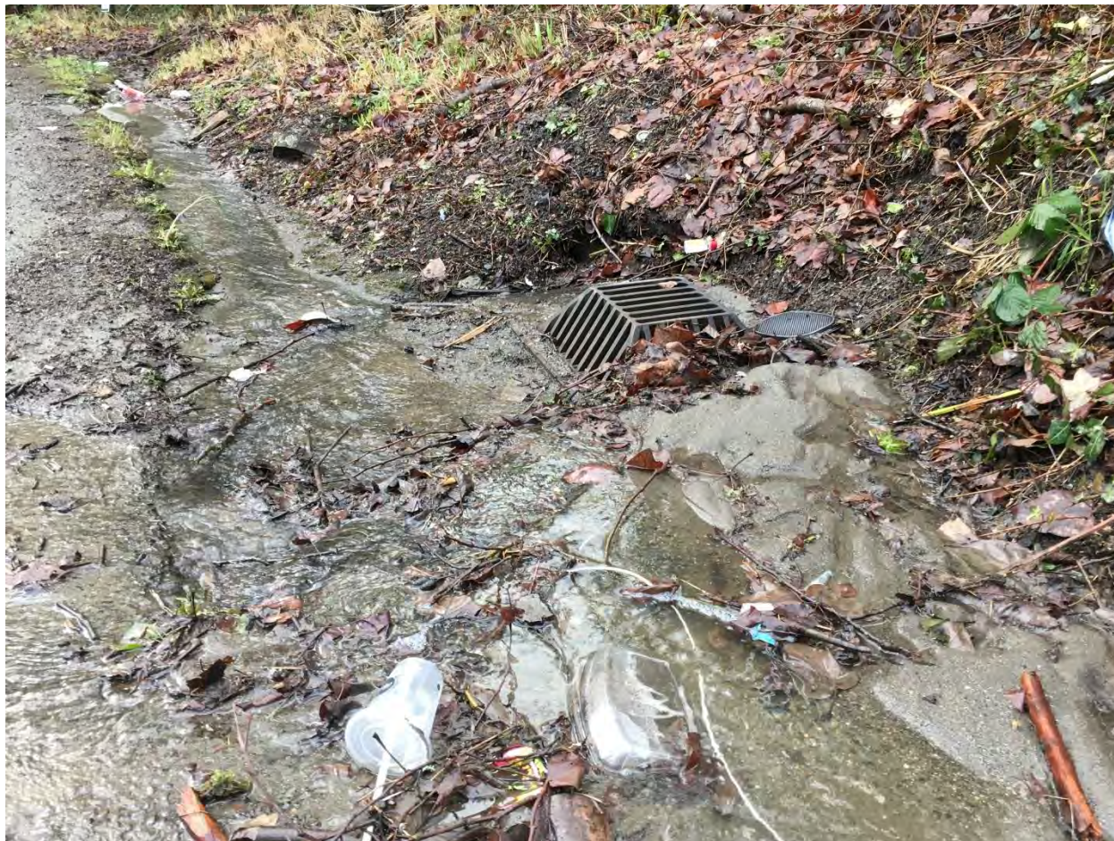
FIGURE 2: Looking south, picture taken 3/12/2019, west side of S 116 th Way, CB11637, flow direction towards south
