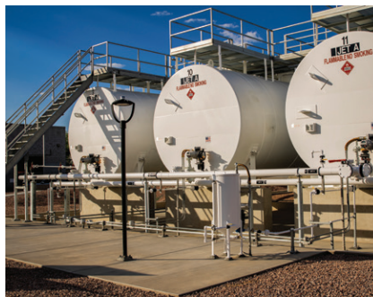
30 Phoenix-Mesa Gateway Boosts Onsite Fuel Storage
