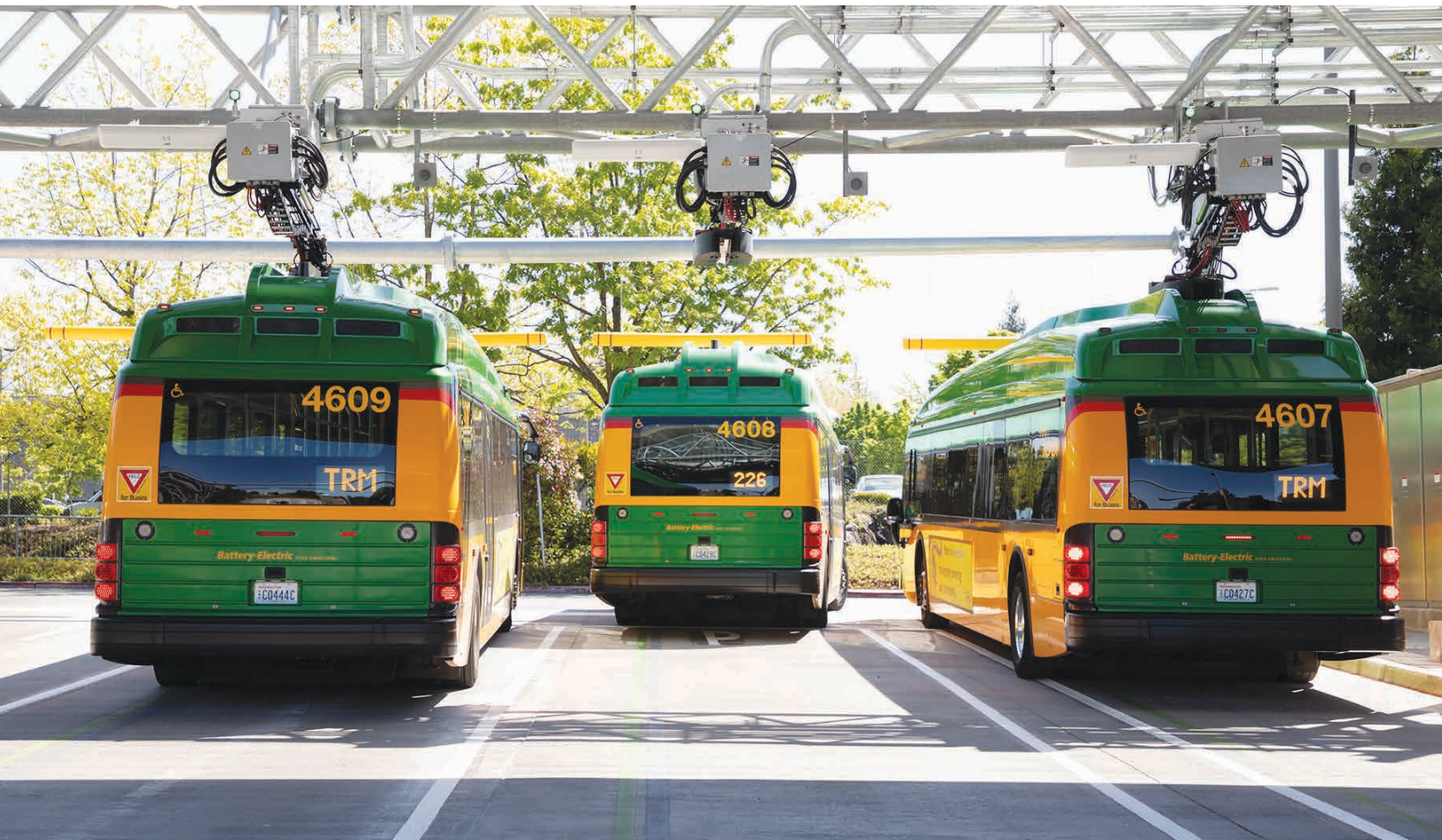
Battery electric buses charging at Eastgate Park-and-Ride.
