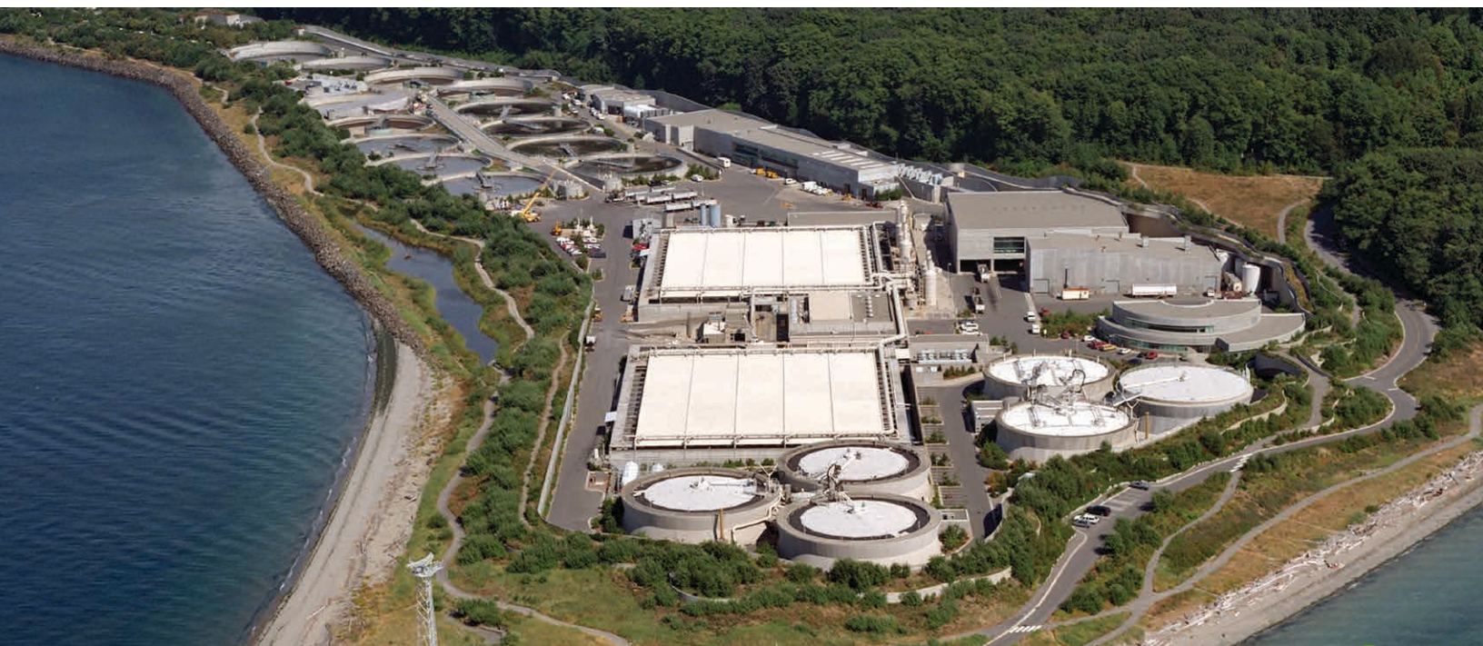
King County's West Point Treatment Plant.
