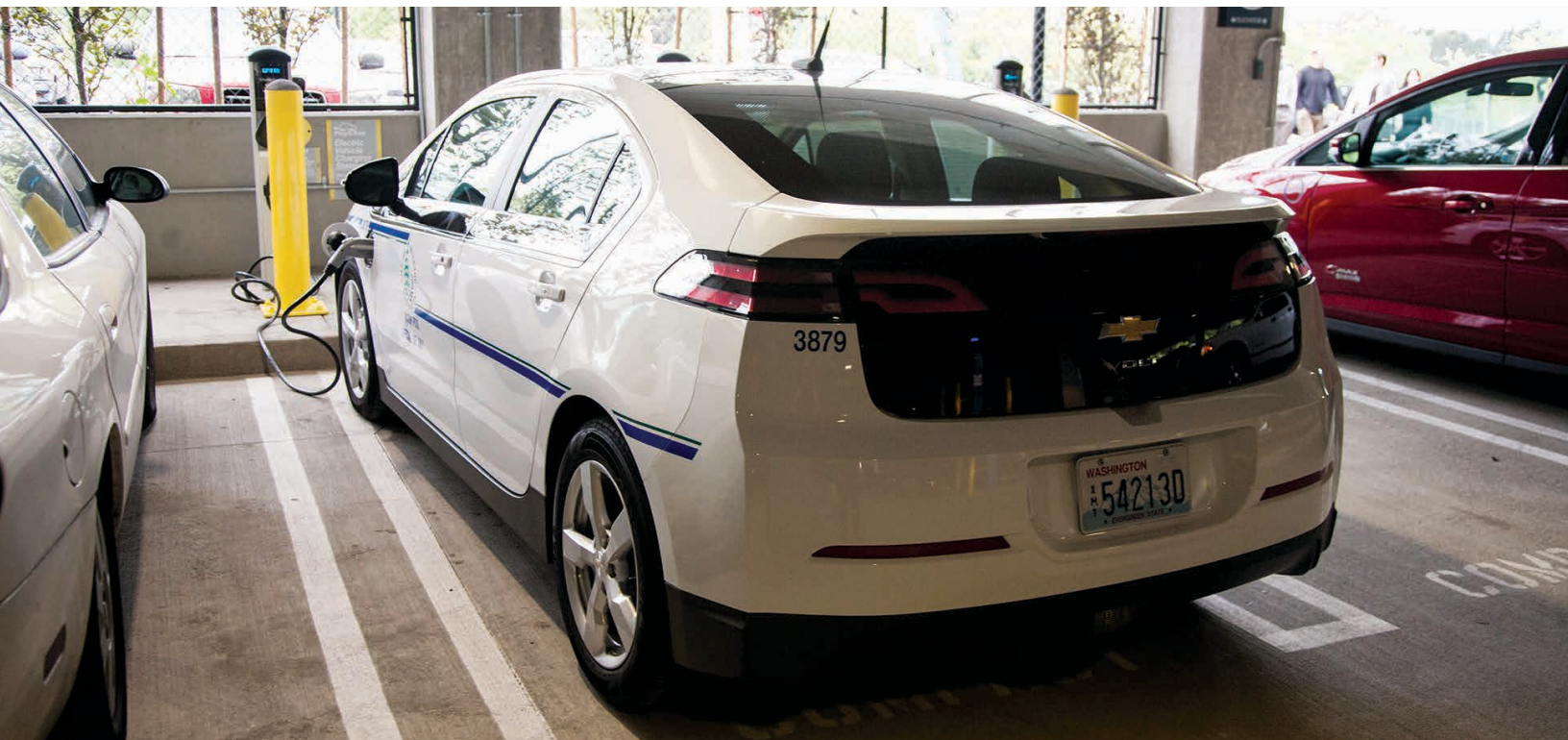
Charging station in use at a King County Park & Ride
