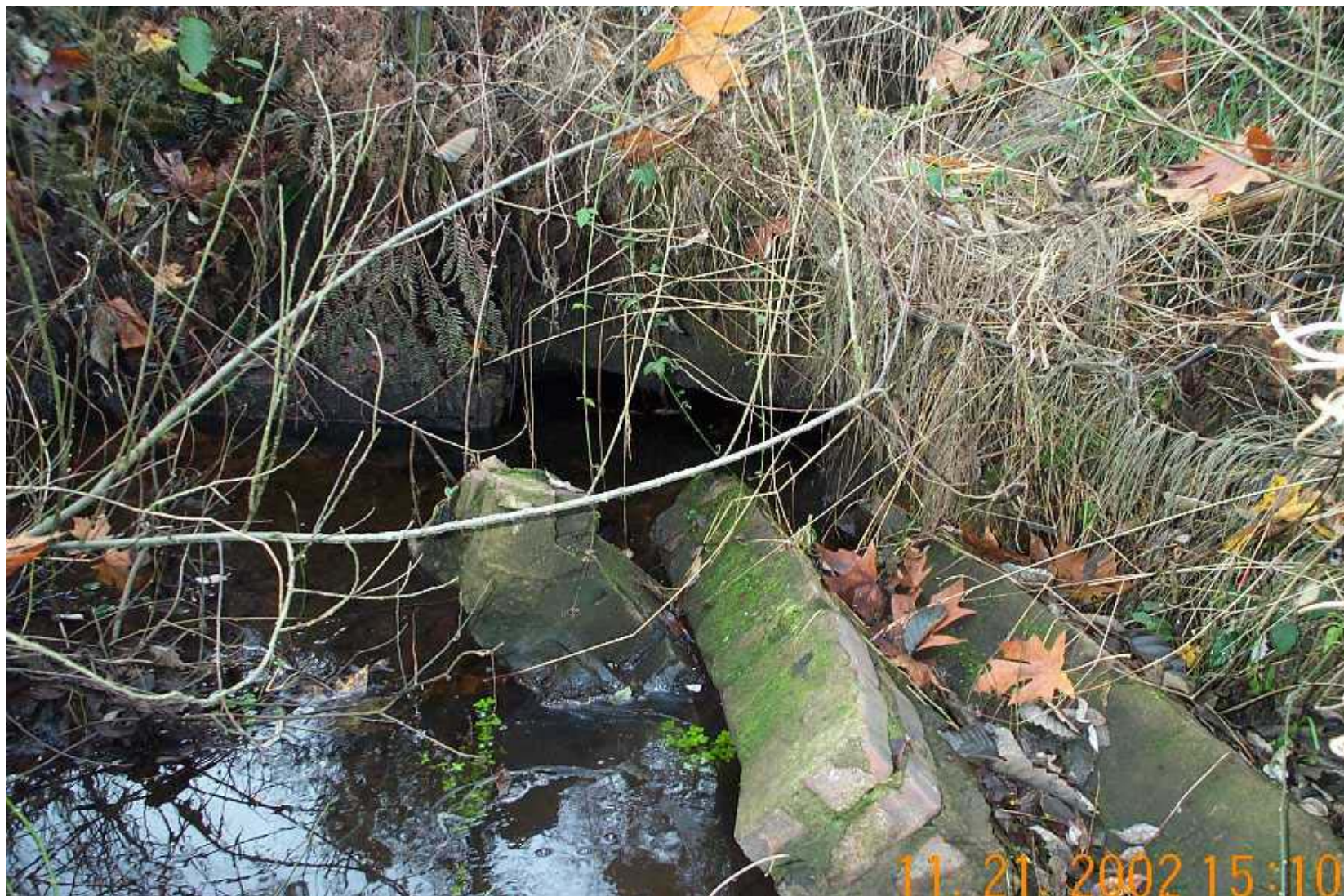
Broken retaining wall along Des Moines Memorial Drive
